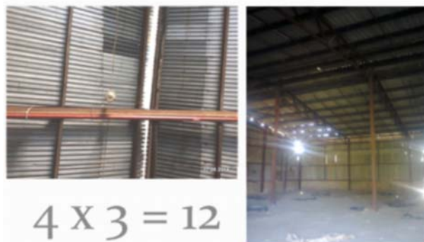
Example : Substantial/Intolerable Risk
